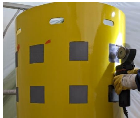
Figure 1: Offshore wind tower mockup structure with predefined repair spots for film application. (Copyright: Muehlhan Holding GmbH)
